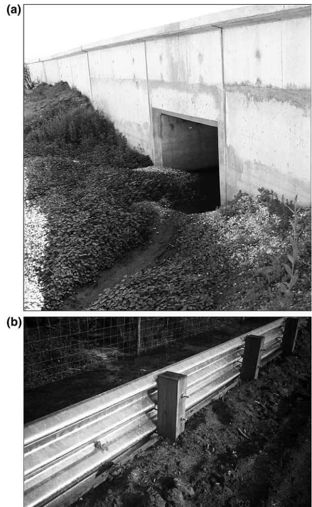
Fig. 1. (a). The barrier wall-culvert system on the northwest side of Paynes Prairie at culvert No. 2. The prefabricated concrete box culvert is 2.7 \times 2.7 m. (b). Type A fence bordering 300 m on the northwest side of US 441 across the prairie basin. This fence was not effective in eliminating trespass.
